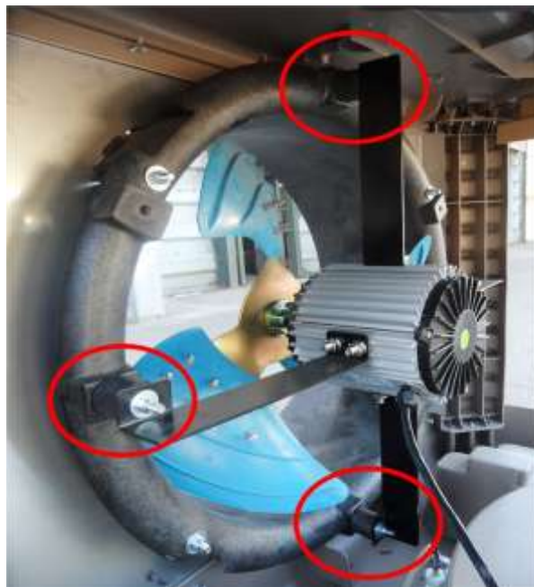
Figure 34. Anti-vibration mounts installed between the motor and the EcoCooler.
